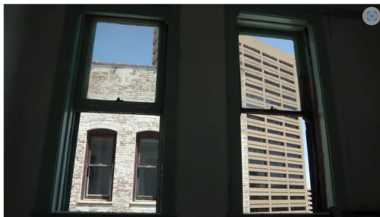
Old wood-framed windows provide views of nearby Downtown El Paso buildings in a room under renovation in the Gateway Hotel at 104 S. Stanton St. RUDY GUTIERREZ/EL PASO TIMES
